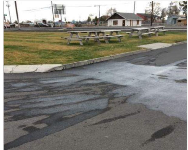
Photograph 4-1. Sewage Overflow in Public Parking Lot
